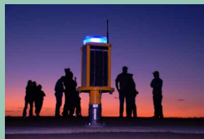
At PMRF, more than 200 solar-powered runway lights were installed to conserve energy.
